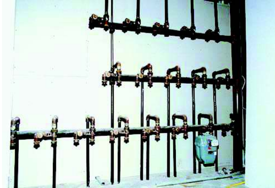
Photo 12. Large Meter Closet
