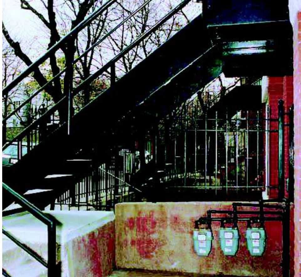
Photo 5. Low-Pressure Service with Outside Riser and Meters
