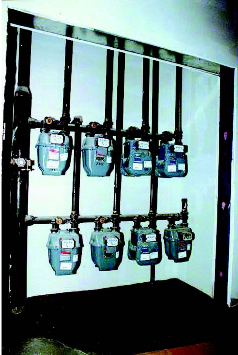
Photo 11. Small Meter Closet
