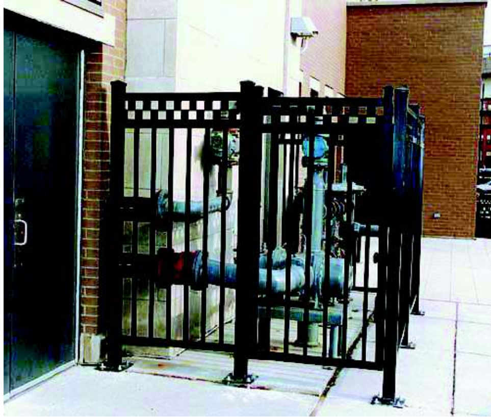
Photo 9. Medium-Pressure Service for Large Volume Installation NOTE: A fence has been erected to protect the large volume regulator station and meter.
