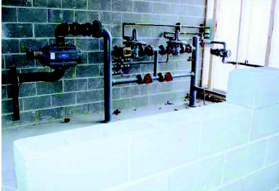
Photo 10. Medium-Pressure Service for Large Volume Installation NOTE: Regulator station and meter have been installed inside within a "Regulator Room".
