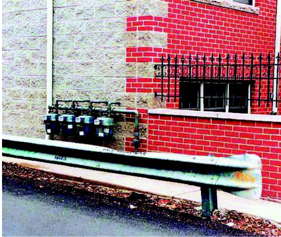
Photo 8. Low-Pressure Service with Outside Riser and Meters Near Alley
