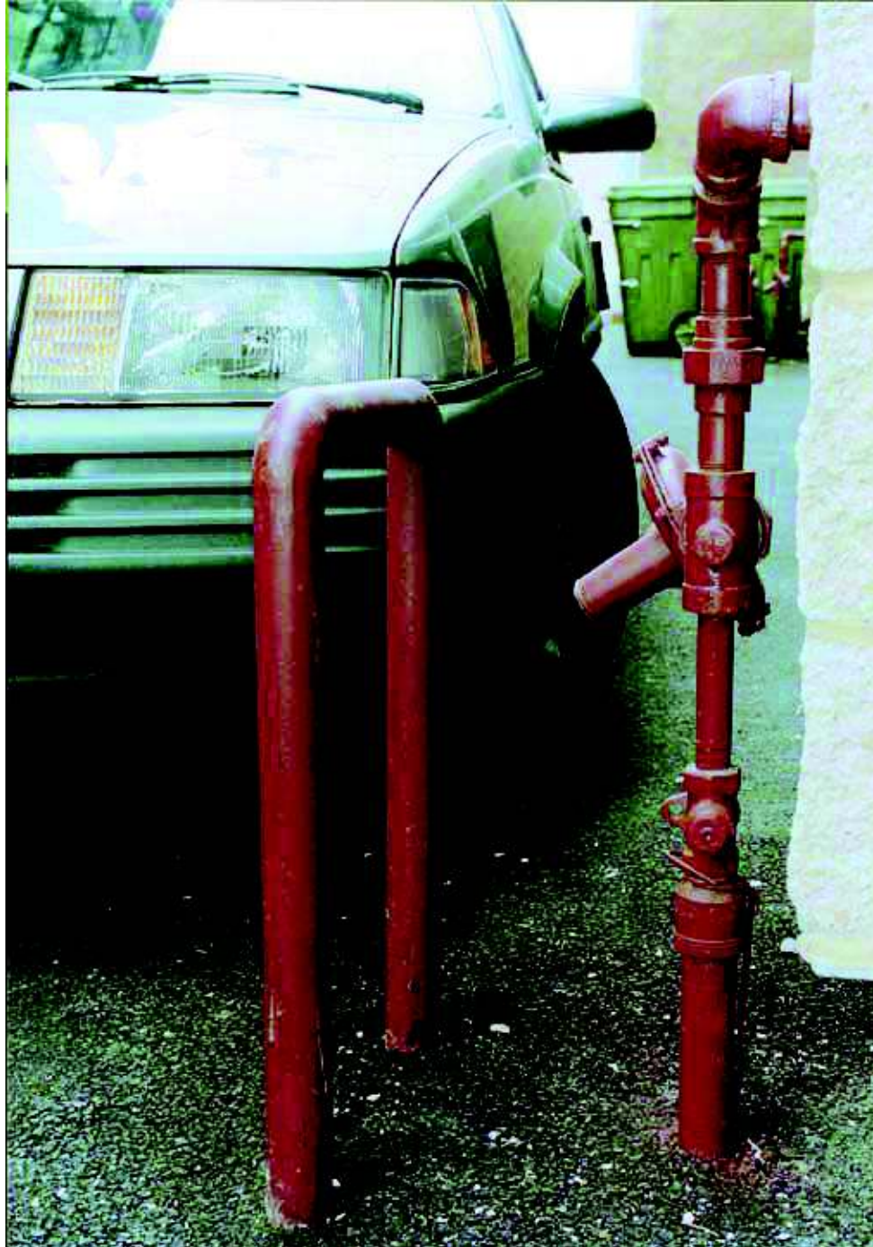
Photo 2. Medium-Pressure Service with Protected Outside Riser NOTE: The service has an outside riser and pressure regulator with a steel "bumper" facing vehicular traffic for protection.
