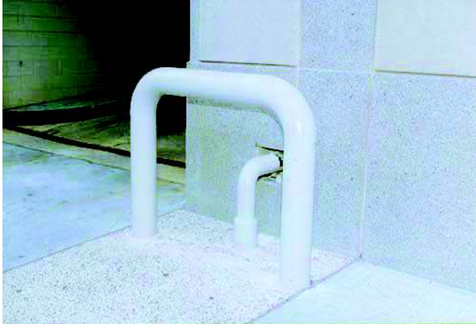
Photo 3. Medium-Pressure Service with Protected Outside Riser and Vents NOTE: The large u-shaped steel “bumper” is used to protect the riser from parking ramp traffic.
