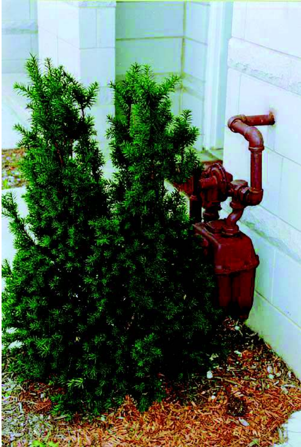
Photo 4. Medium-Pressure Service with Hidden Riser, Regulator and Meter NOTE: The entire service has been installed at the front of the building and has been hidden from view by the installation of small bush.
