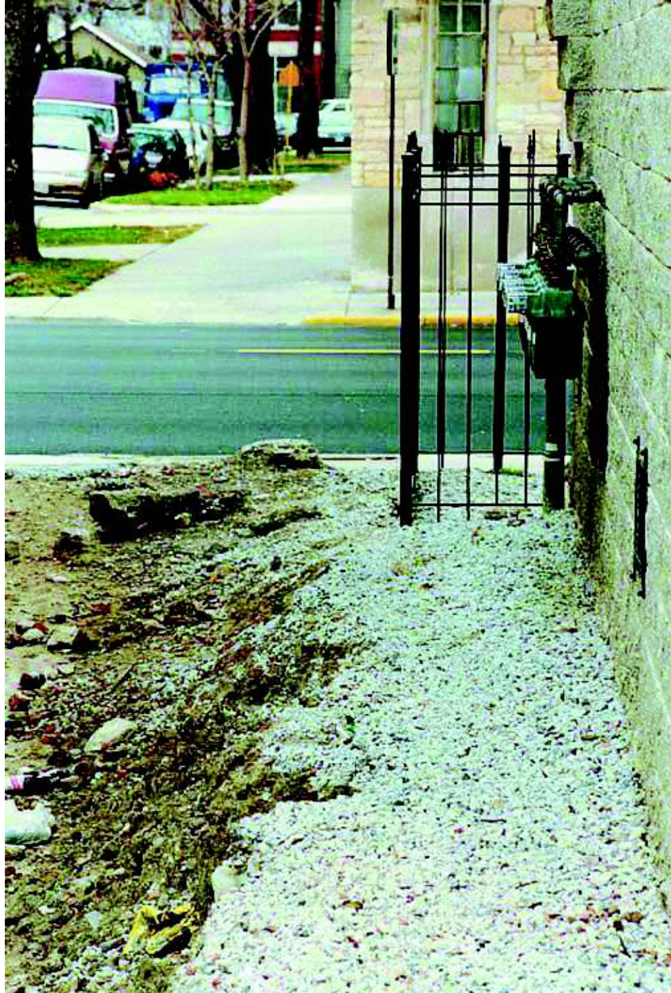
Photo 7. Low-Pressure Service with Outside Riser and Meters
