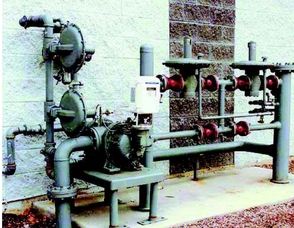
Photo 6. Medium-Pressure Service for Large Volume
